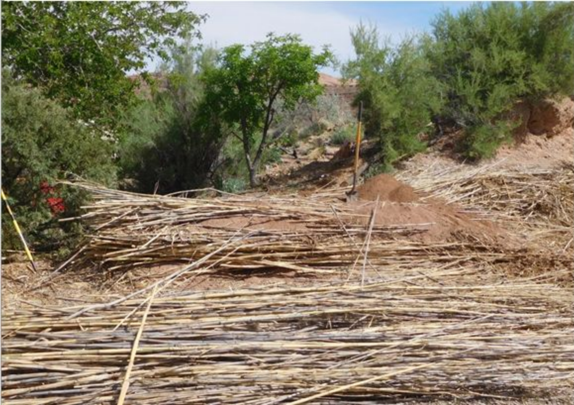
Figure 37: Building the structure in lifts of organic and mineral materials increases bulk density and stability of the structure, allowing for more rapid vegetation.
