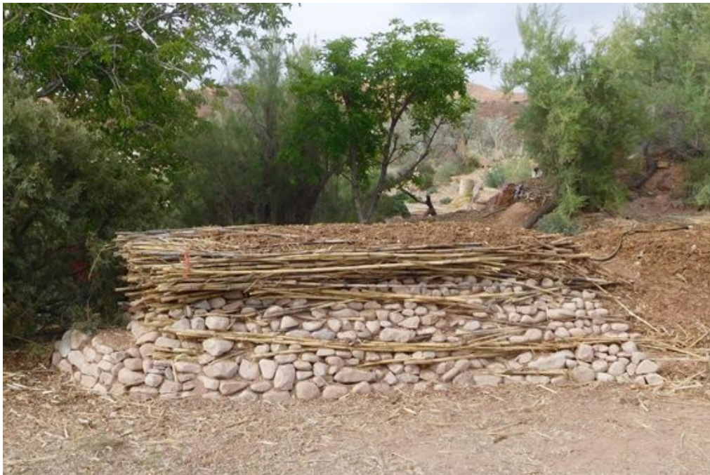
Figure 38: Rock armoring was added to further stabilize the structure and provide for an aesthetic finish.
