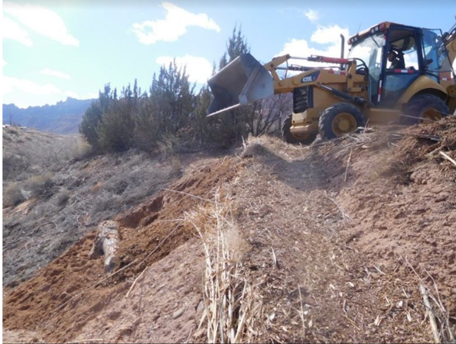
Figure 5: In the early stages of this path system a backhoe was used to anchor large logs into the hillslope and deposit bulking materials. This log is now covered in 10-15 feet of material and the flat top access is protruding 30-40 feet out from the original top of slope.
