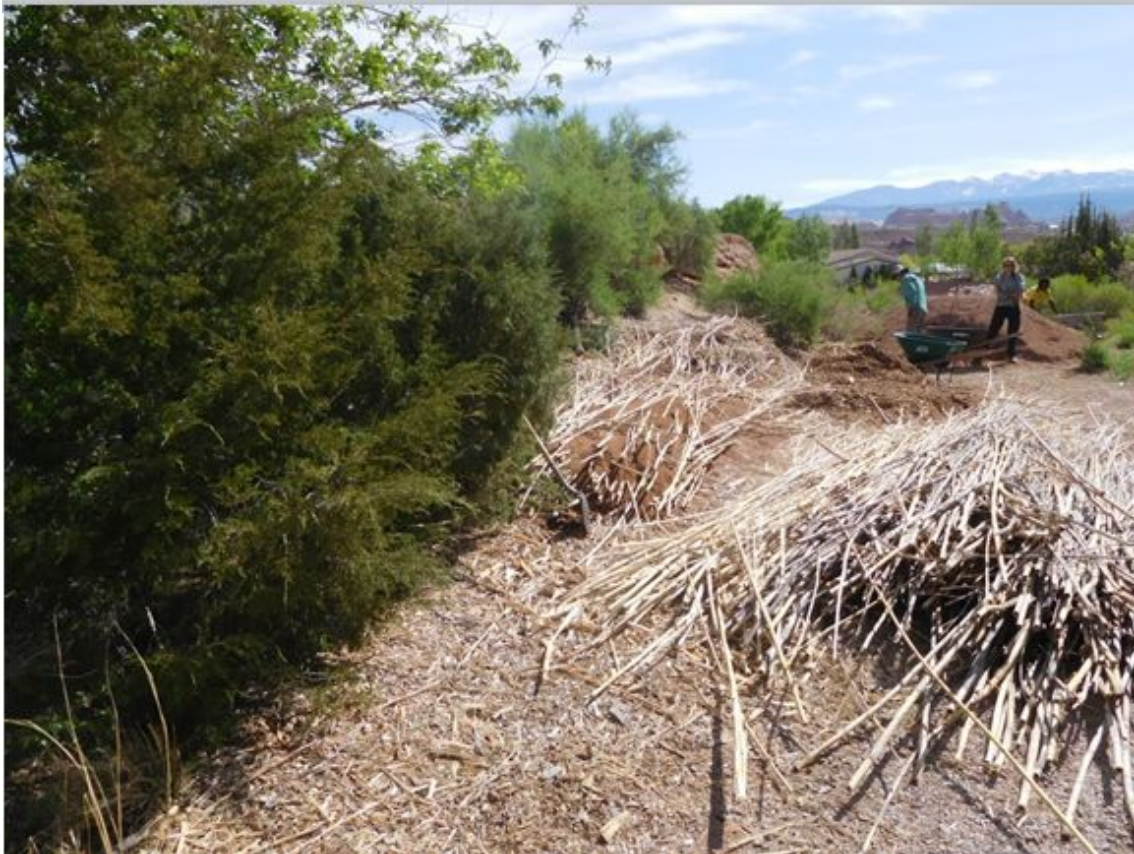
Figure 36: Procuring and staging materials close to the structure makes building more efficient.
