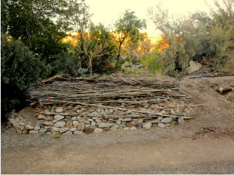
Figure 40: A diverse seed mix was used to establish vegetation on top of this berm.
