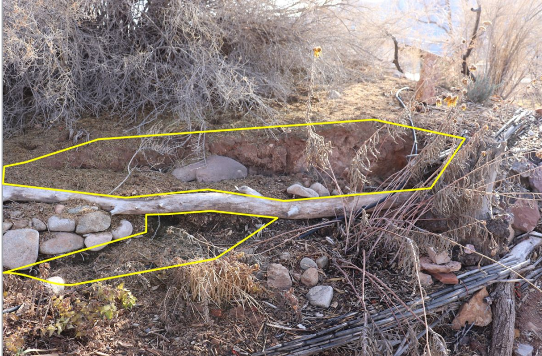
Figure 33: Brush-mineral structures that are not implemented with a high bulk density are more prone to settling and may be difficult to establish plants on. Low bulk density areas are settling above and below the horizontal log (yellow outline), while vegetation has been established just below these areas due to increased mineral soils added to the layers.
